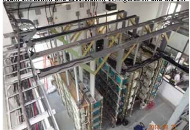
Figure A.2.7.1 Power Supplies installed for Negative Ion Beam Source Experiments
