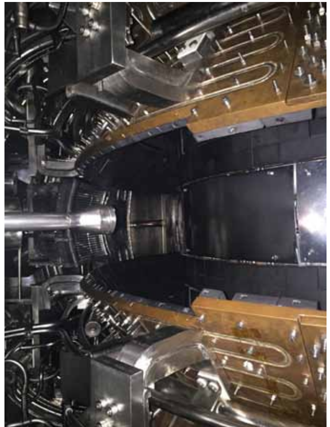
Figure A.1.2.3 SST-1 up-gradation is going on with plasma facing components
