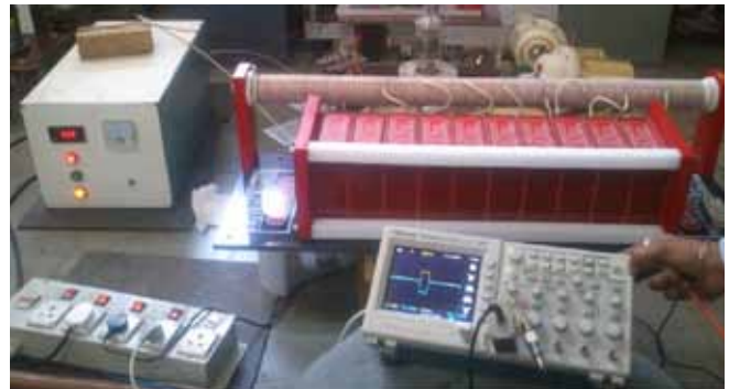
Figure A.3.4.1 The Pulsed Modulator System being developed
