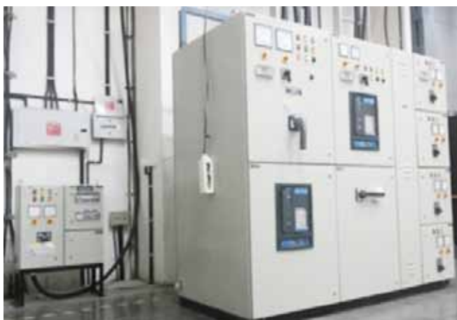
Figure A.2.7.2 Control panel for Power Supplies
